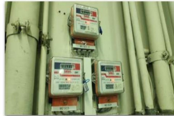
Electrical sub-meters installed at Royal Duty Free Shops
